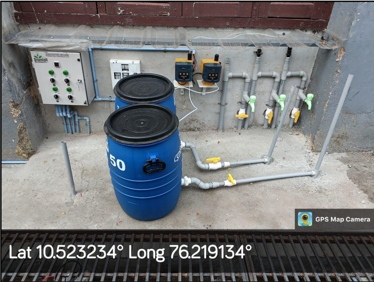
Waste Water Recycling Plant in Science Block
