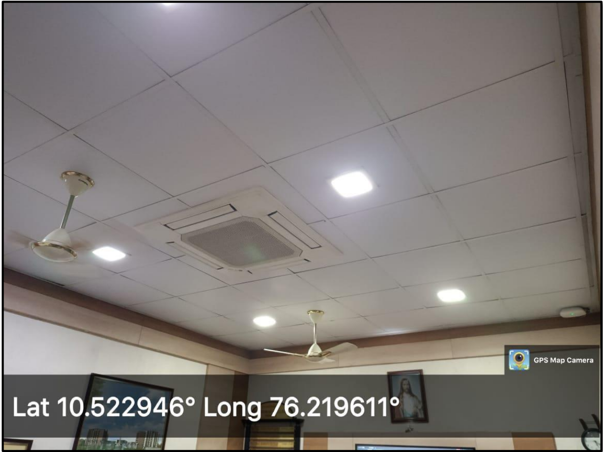
Daikin VRV IDU High Walls at Principals Room
