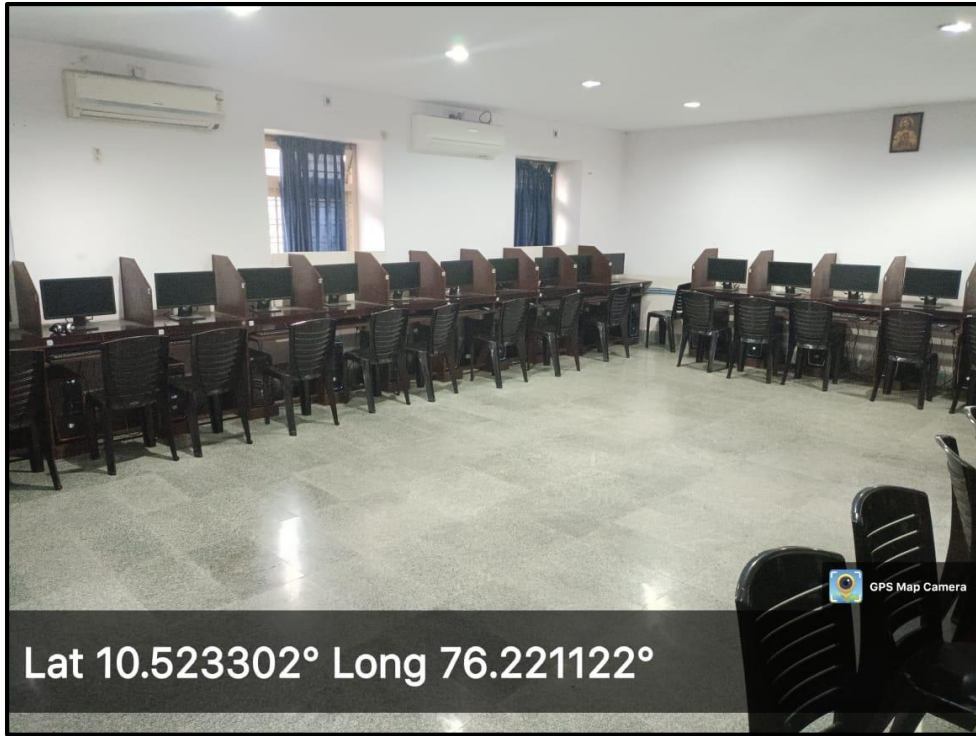
LED lights in Electronics Lab Jubilee Block
