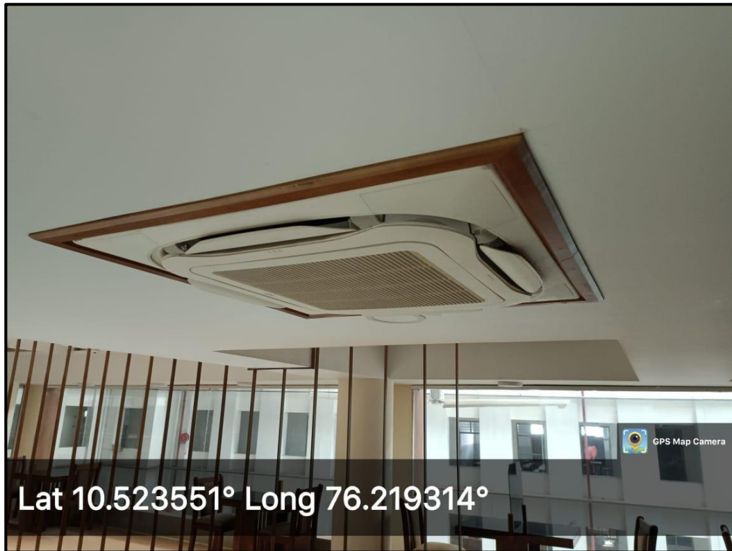
Daikin VRV IDU High Walls at Library
