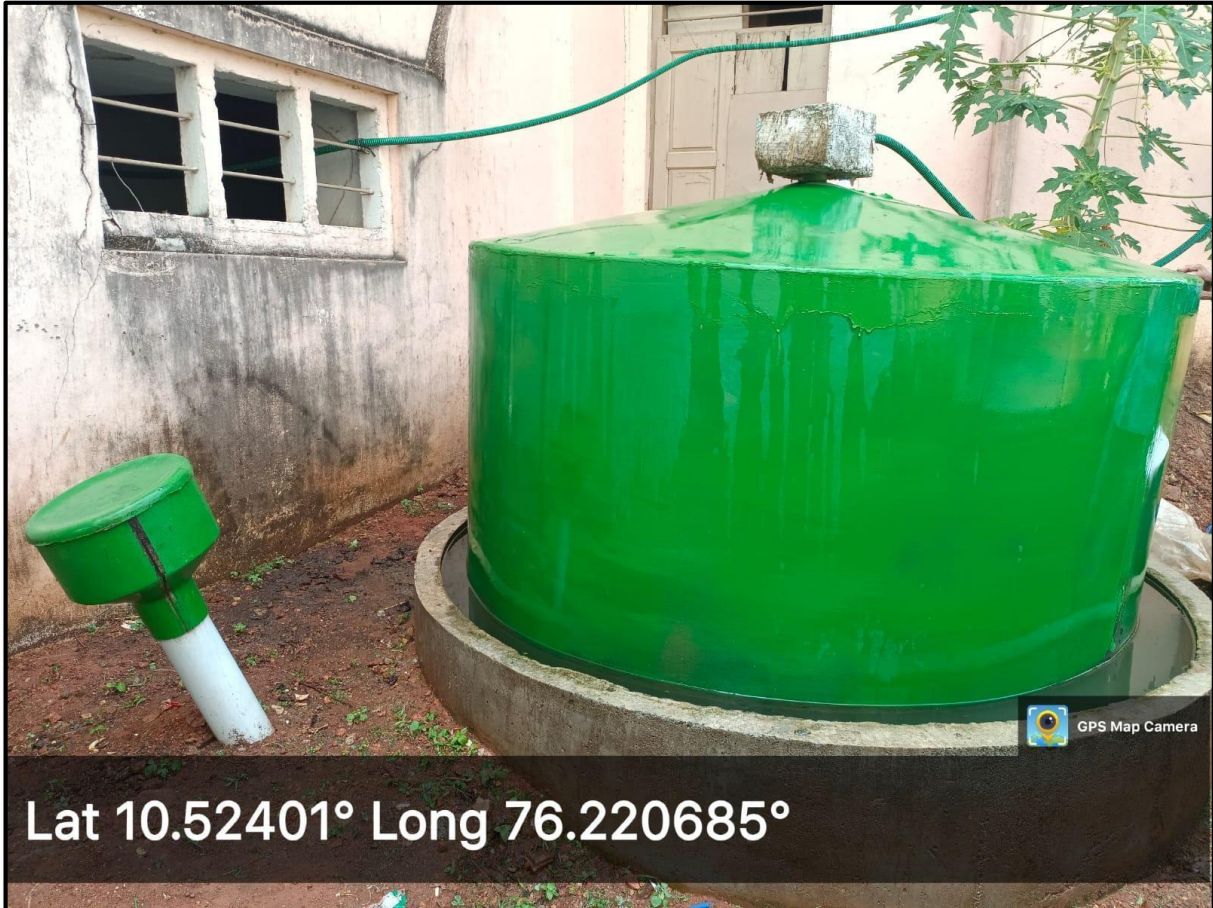
Bio Gas Plant in the Hostel
