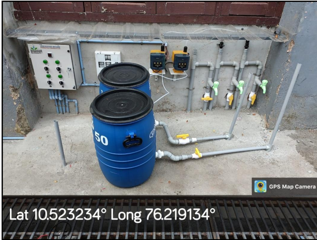
Waste Water Treatment Plant near Science Laboratories
