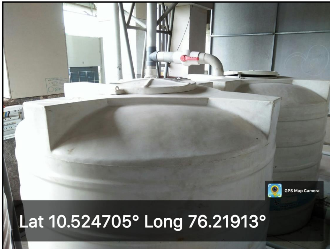
Rain Water Collecting Tanks at Academic Block
