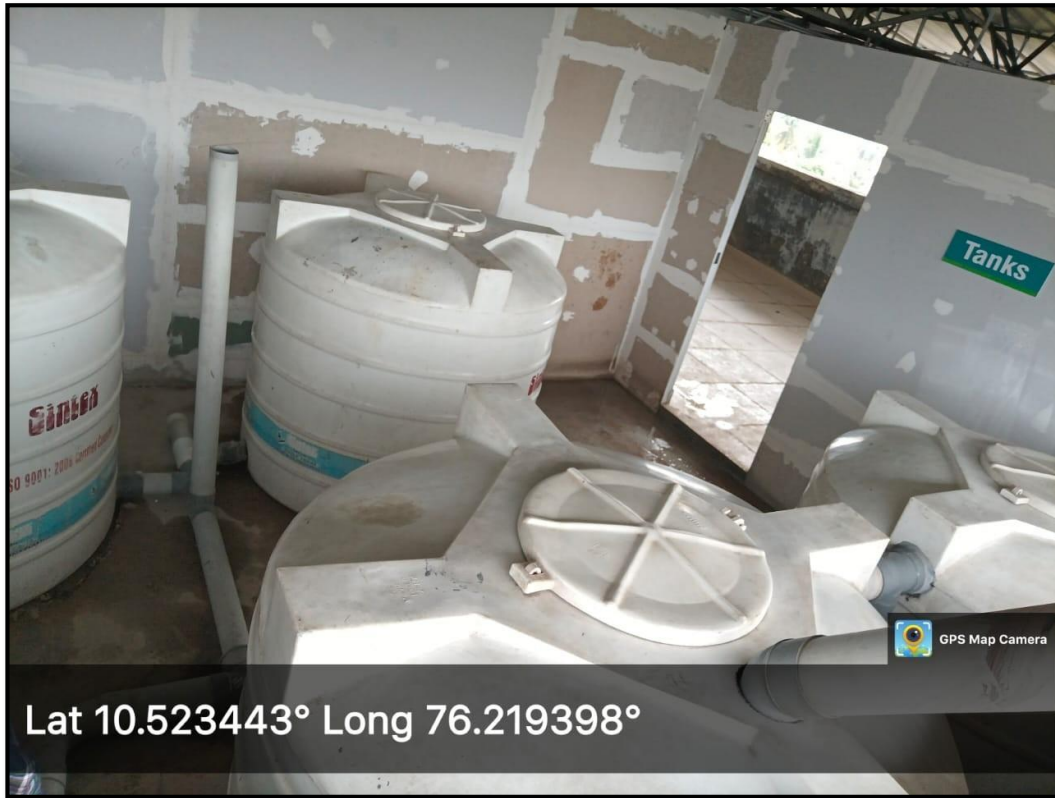
Rain Water Collecting Tanks at Academic Block
