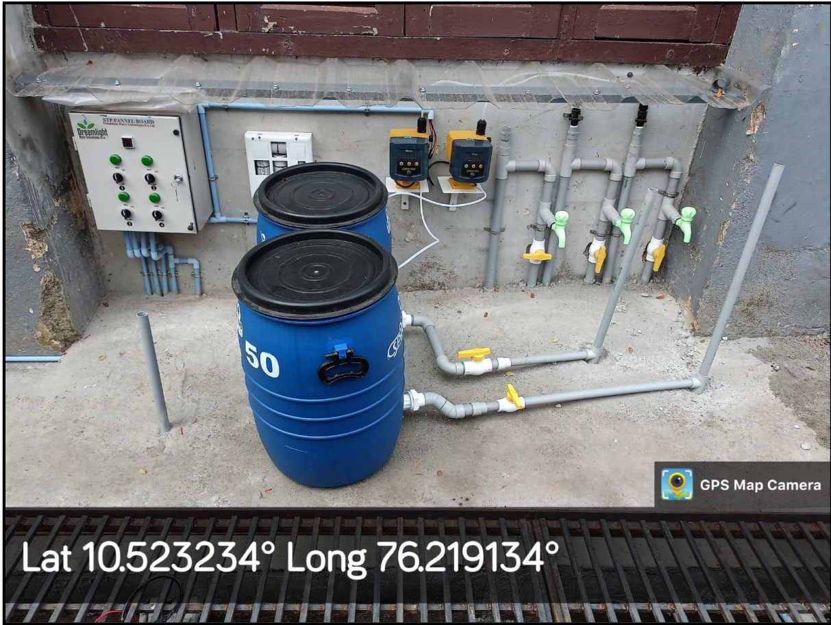
Waste Water Recycling Plant in Science Block
