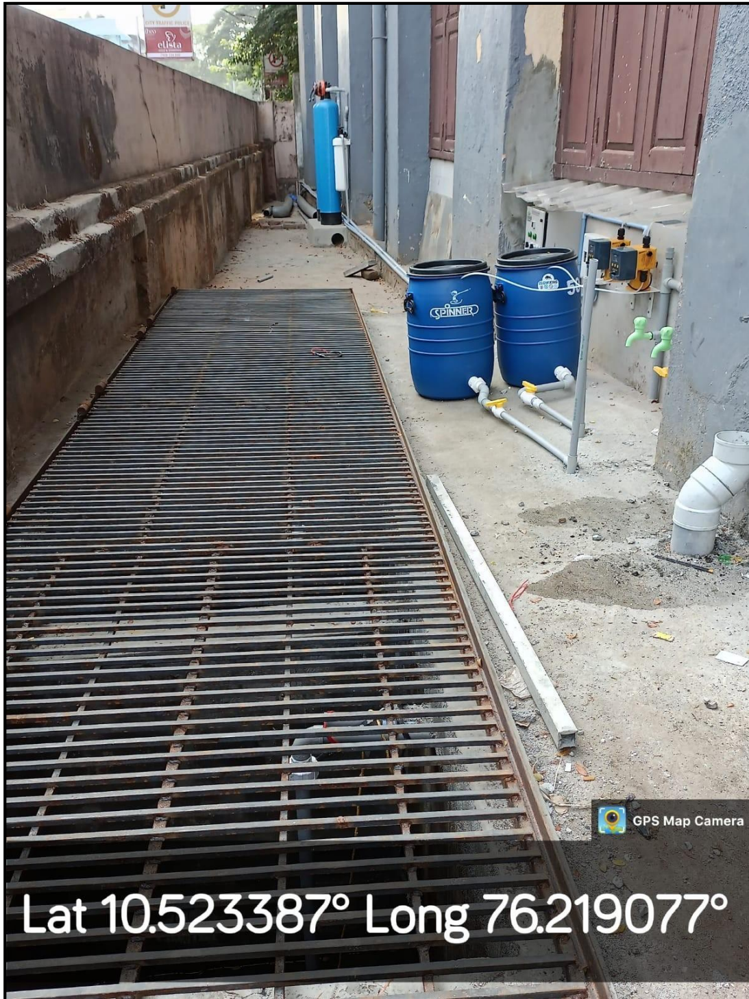
Waste Water Recycling Plant in Science Block
