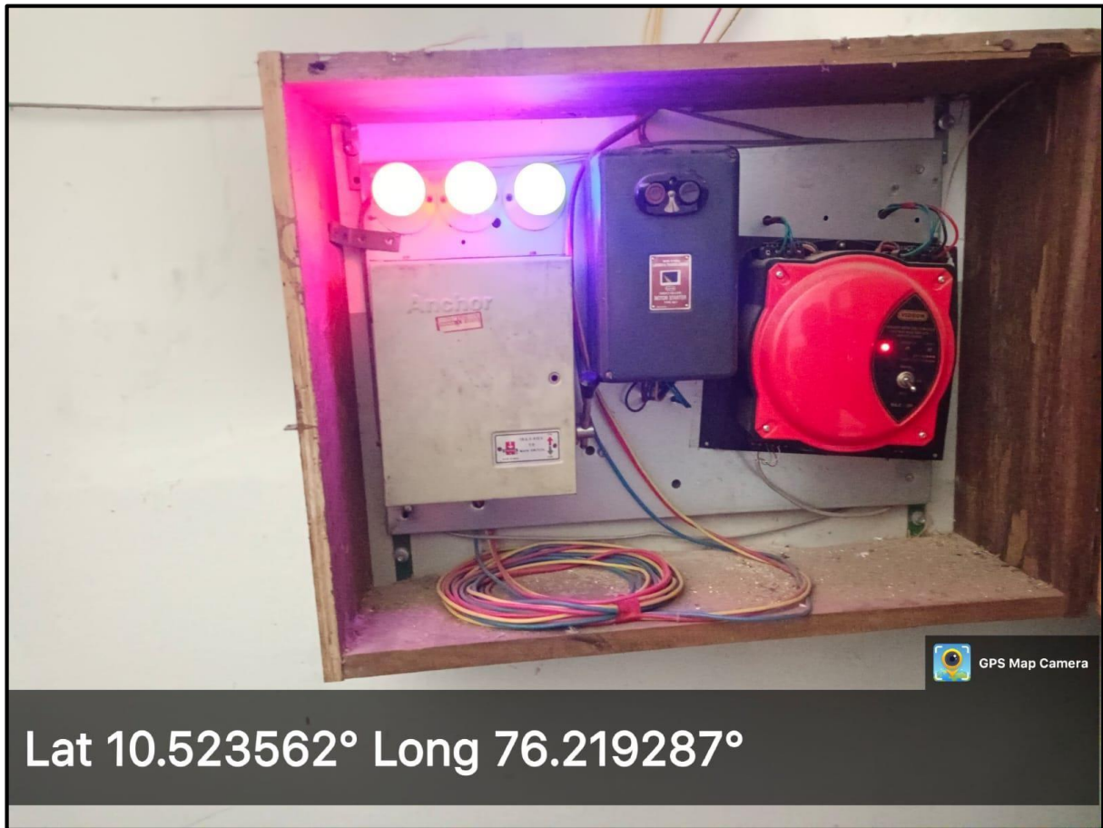
Fully Automatic Water Tank Level Controller at Academic Block
