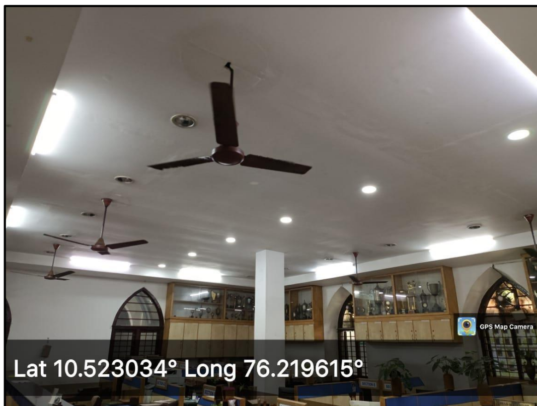
LED lights in College Office
