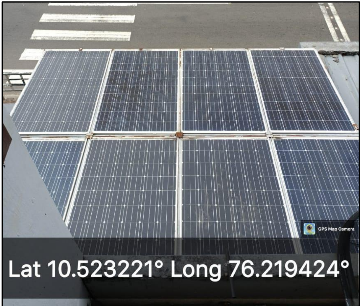
Solar Panel of 5 KV Placed on above the Canteen
