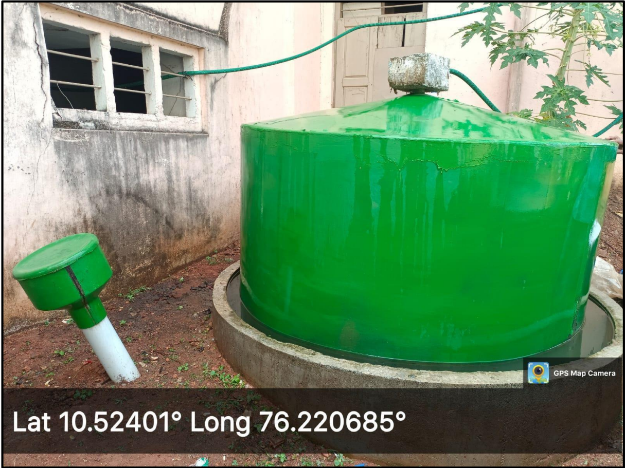
Bio Gas Plant in the Hostel
