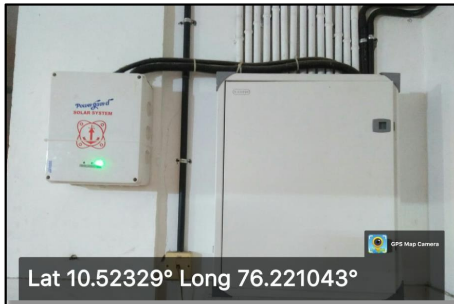
Solar System In Hostel
