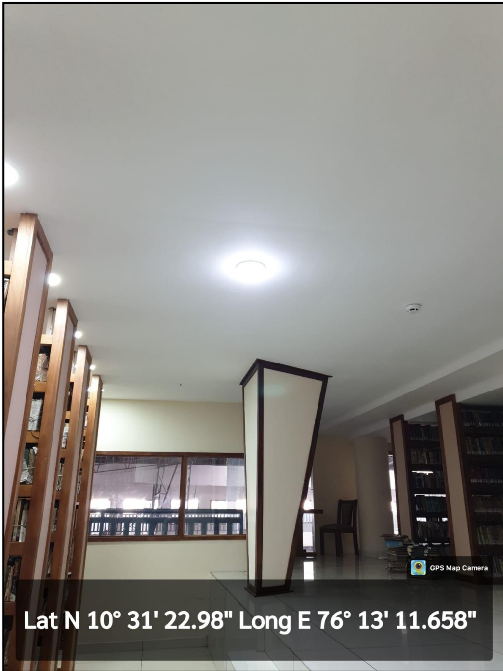
Sensor Light and Smoke Detector In Library
